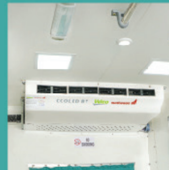
Powerful air-conditioning unit
